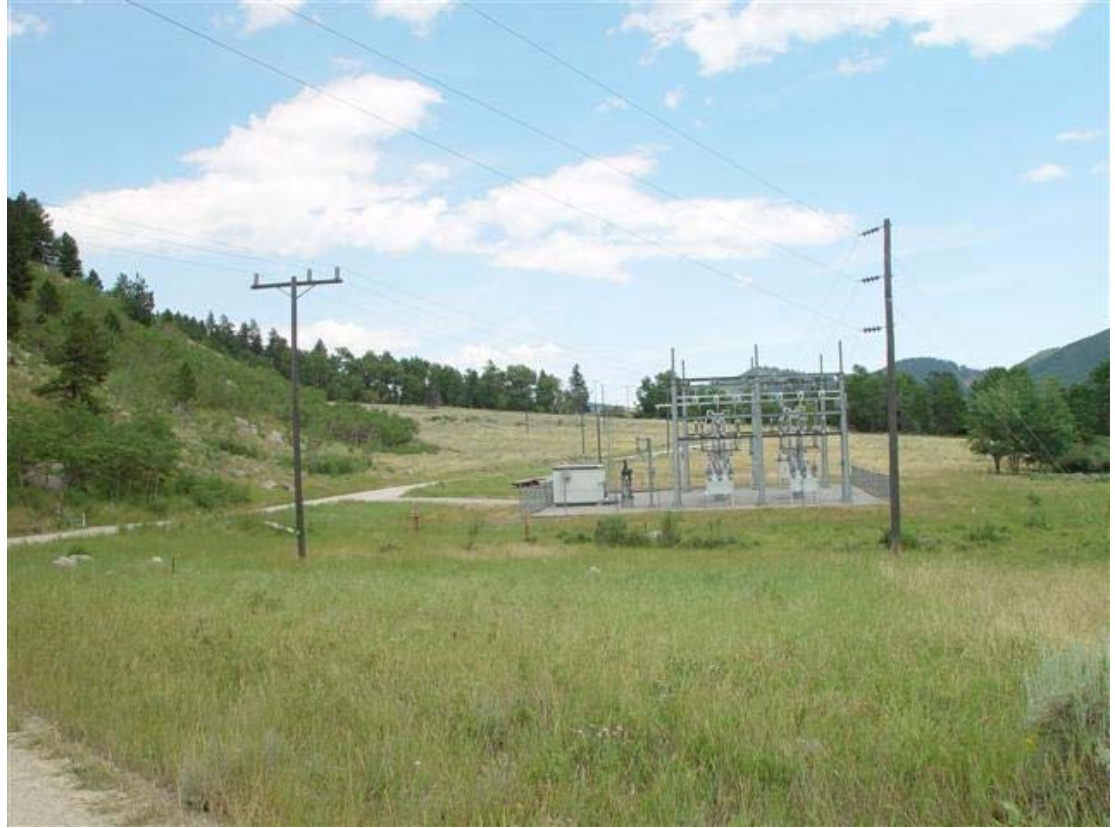
Figure 3. Line Creek Substation
